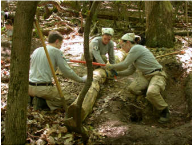
The park's popular trail system needs regular maintenance. Much of the work is provided by volunteers, such as this Americorps crew.
