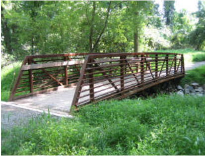
Replacing deteriorated infrastructure, such as this River Trail bridge, is typical of needed investments.
